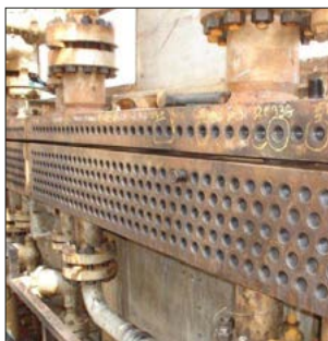
FinFan cooler before a maintenance
